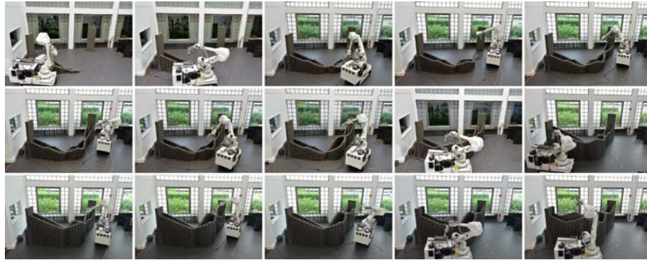
Fig. 9. Images taken from a time lapse video of the building process. The whole video is viewable at: https://youtu.be/loFSmJO3Hhk .
