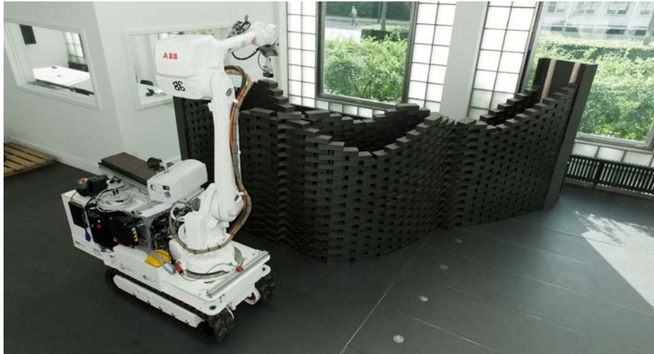
Fig. 10. Experimental result: Double leaf dry stacked brick wall fabricated by the mobile robot. (Photographer: Michael Lyrenmann)
